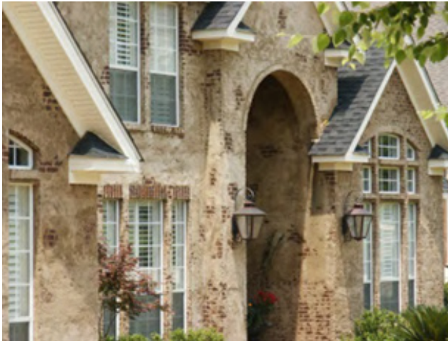
Photo 6 Mortar Wash Obscuring Areas of Brick
